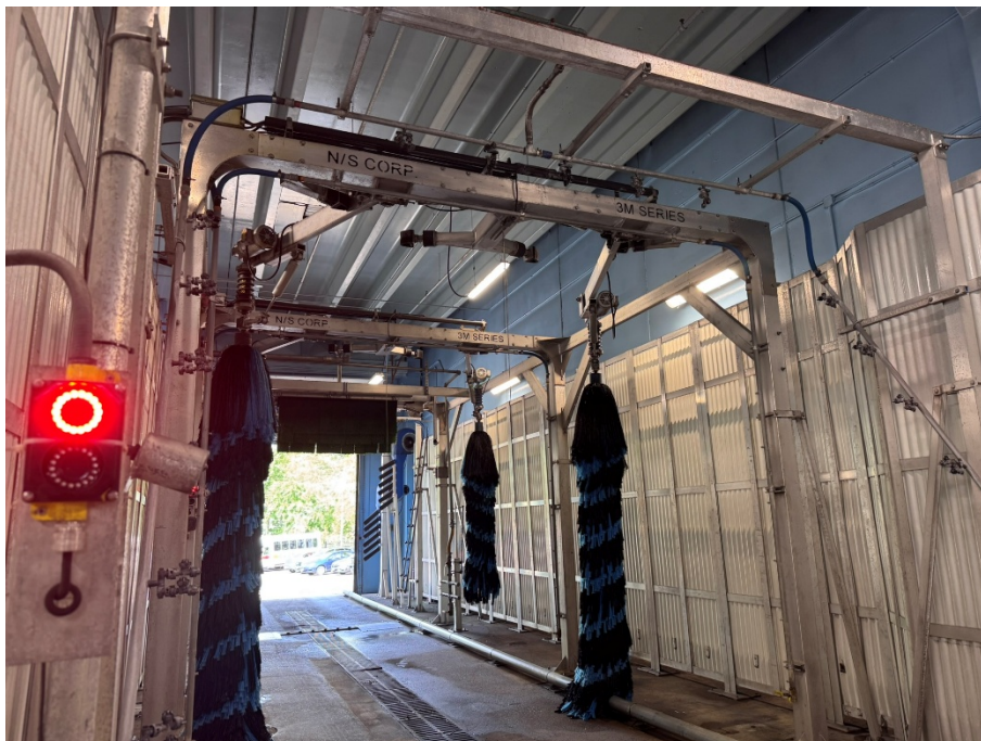
ARCH-12: RECENTLY UPDATED BUS WASH EQUIPMENT
