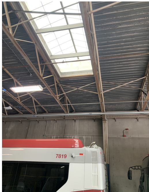
STRU-04: TYPICAL CONDITION AT UNDERSIDE OF THE METAL ROOF DECK AT THE MAINTNEANCE AND BUS STORAGE AREAS
