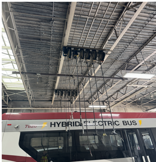
EQUIP-01: FLUID DISTRIBUTION REEL BANKS
