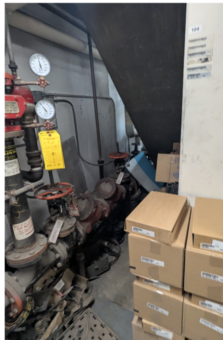
FP-01: SPRINKLER BACKFLOW UNDER STAIRS
